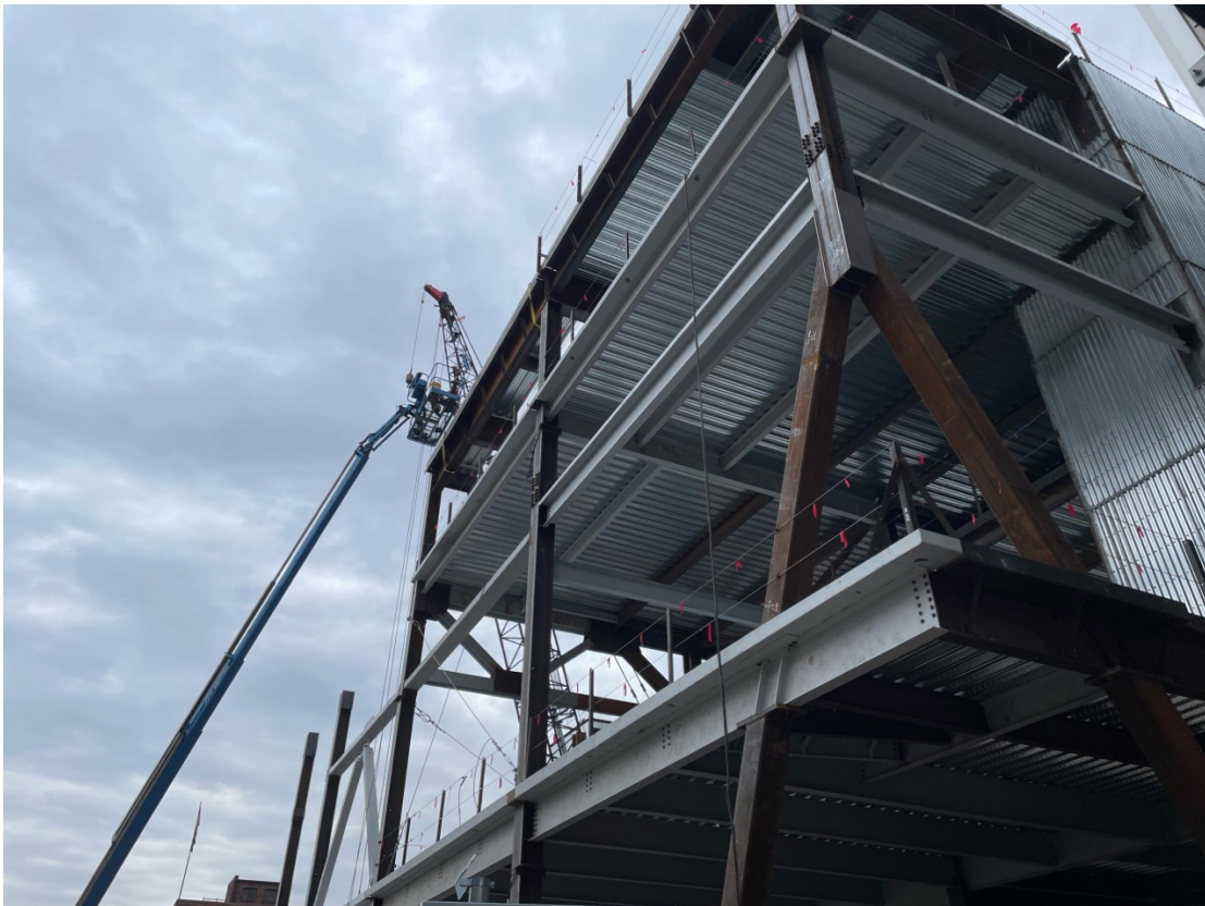
Visitors to downtown Ithaca can see construction progress for the new conference center. (Photo by: Jillian Bleier/Ithaca Week)
