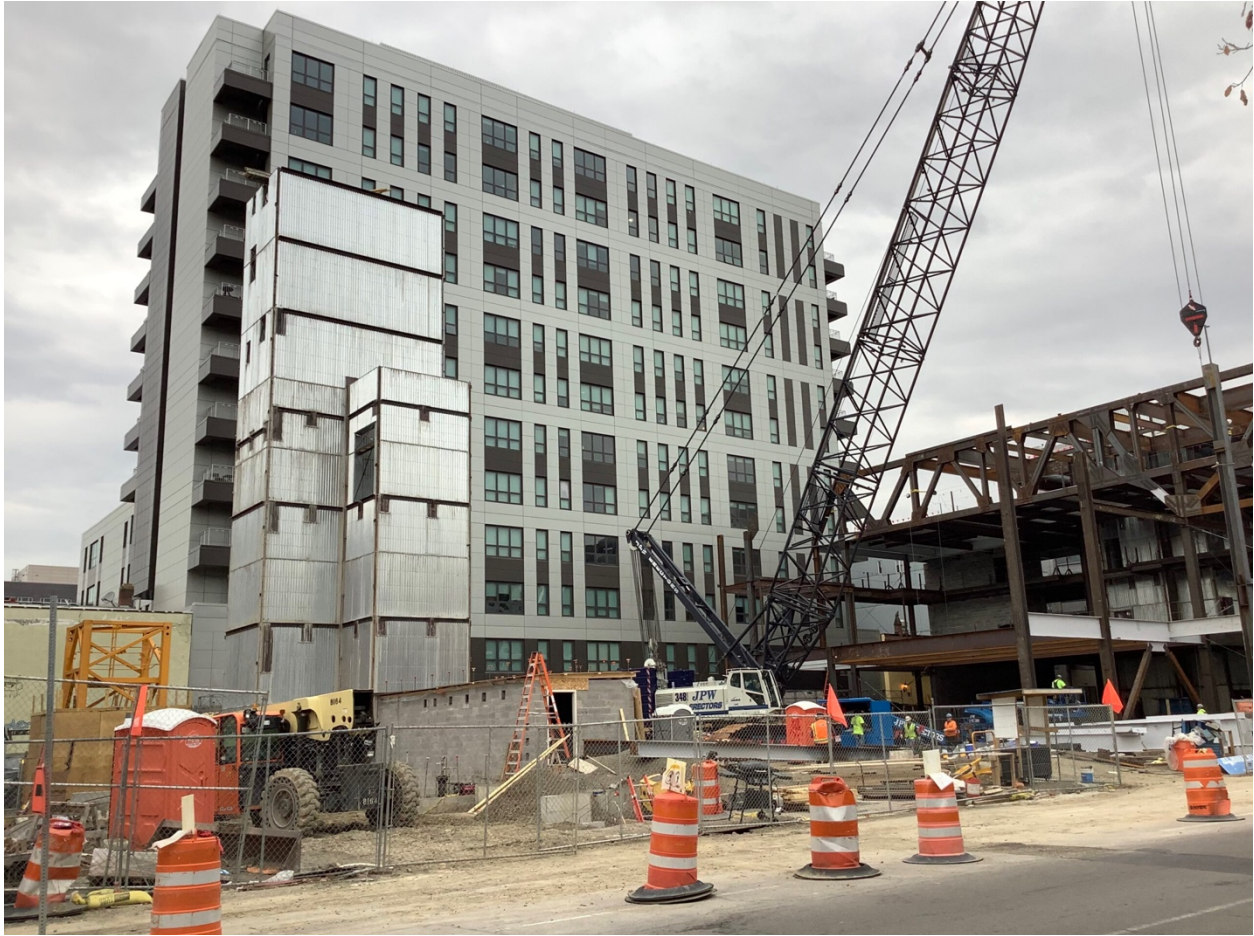
Construction above ground is making progress. Elevator shafts are being built for the building, as well as other structural components. (Photo by: Jillian Bleier/Ithaca Week)
